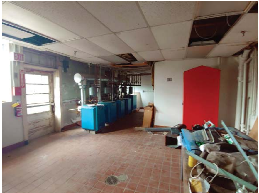
Ground Floor - Utilities Room, Heating System.
